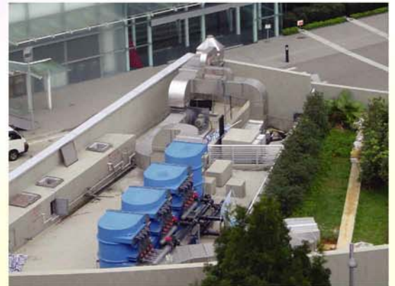
Water Scrubber for Refrigerant Leakage Protection
